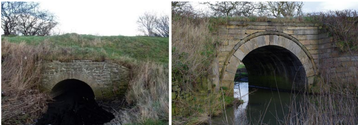
Plate 17. Oakley Beck and Hummerbeck culverts – both original 1825 structures but with differing degrees of architectural ornamentation
