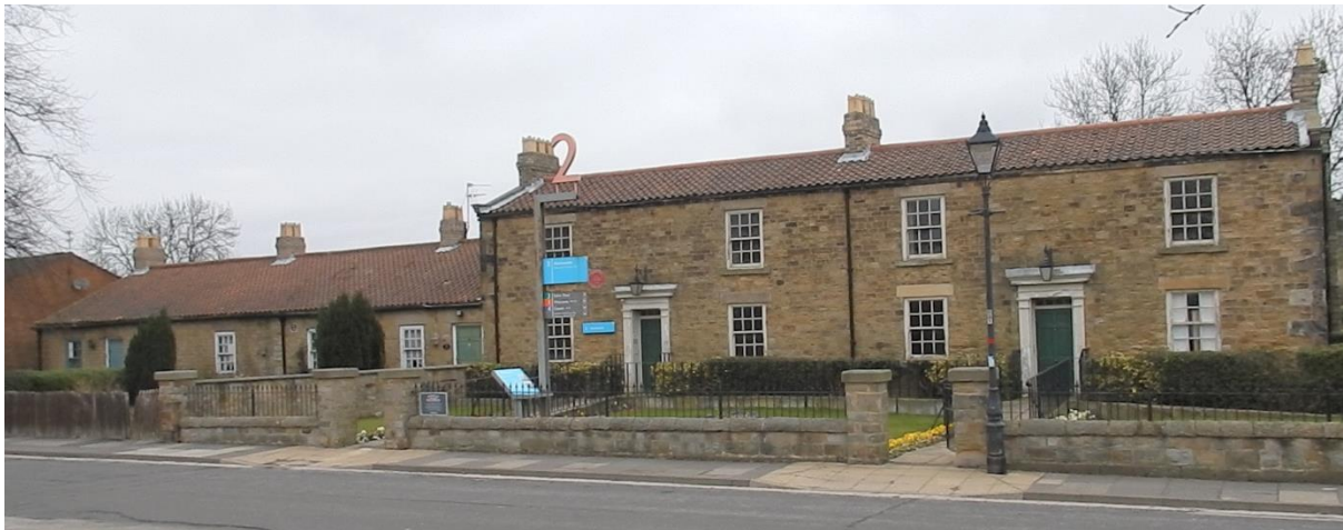
Plate 12. Soho Cottages. Having been rescued in 1974, they are now in a state of disrepair with broken windows and rotting window frames. Their future uses need serious consideration including their role in generating additional income for the museum. The Hackworth family had their own garden, grew their own vegetables and had a little livestock (Young 1975, 182). The gardens are therefore also potential locations for community excavation with scope to return the gardens back to a representation of their 1833-50 condition.
