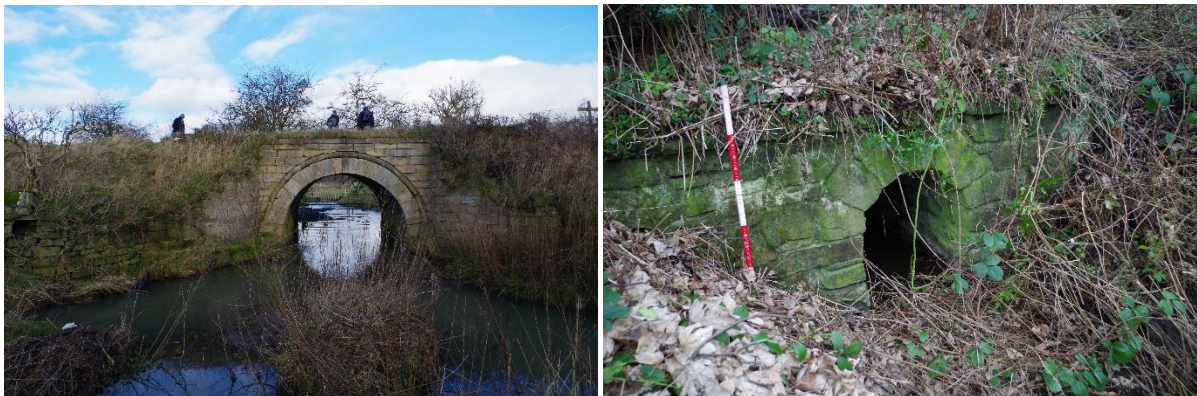
Plate 5. Left: The Hummerbeck Bridge with typical string coursing to the arch. It also had peppercorn terminals which have fallen off but lie nearby. Right: a culvert below Etherley Incline
