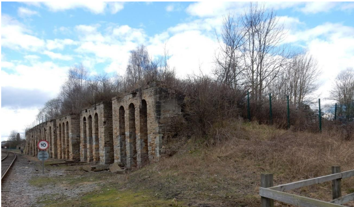
Plate 11. The coal drops in 2016. These are now in desperate need of conservation.
