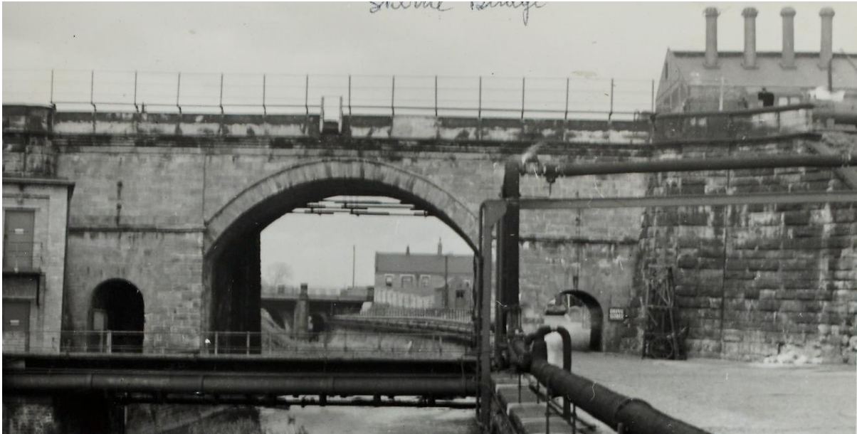
Plate 18. The Skerne Bridge in the 1950s. Photo from the Bibby Collection in Durham University's Special Collections. Unaccessioned.
