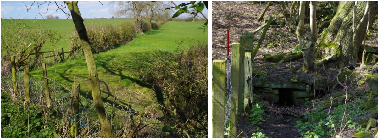
Plate 14. The incline has a crossing point consisting of metalled earth ramps to east (above left) and west. The drainage ditches of the incline run beneath the ramp in stone culverts (above right)
