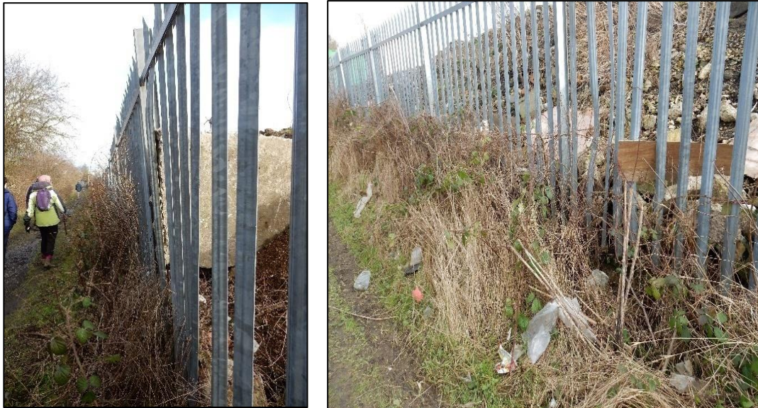
Plate 20. Scrap yard, unattractive boundary, spillage and litter
