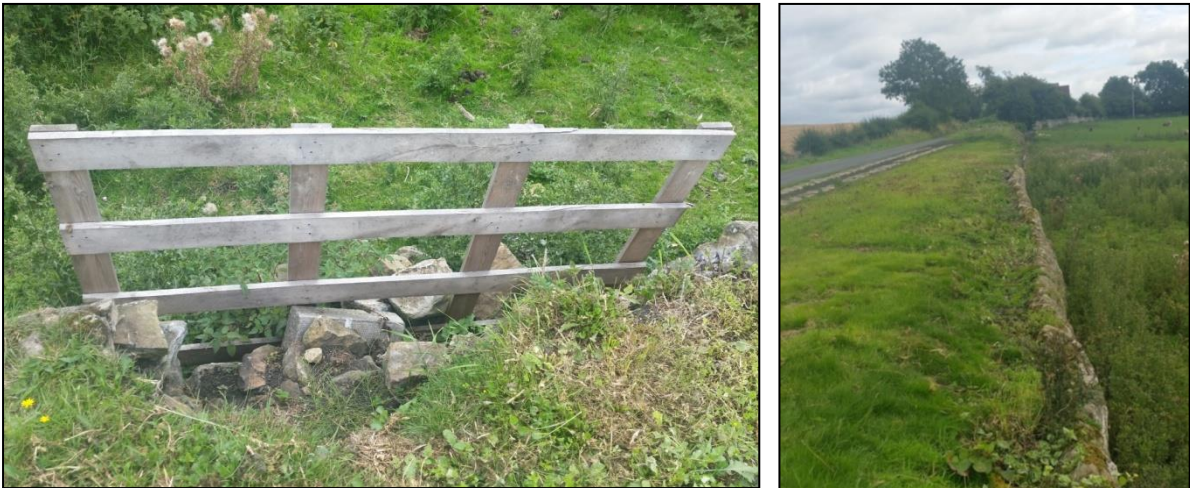
Plate 13. The boundary walls of the Brusselton Incline embankment also act as retaining structures. The north side was repaired in the early 1990's but the south side and localised areas are also in need of repair all the way to the top and the reservoir.
