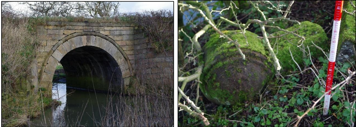
Plate 5. Hummerbeck Bridge (south side) and fragments of the north side of the bridge parapet knocked over and lying amongst vegetation
