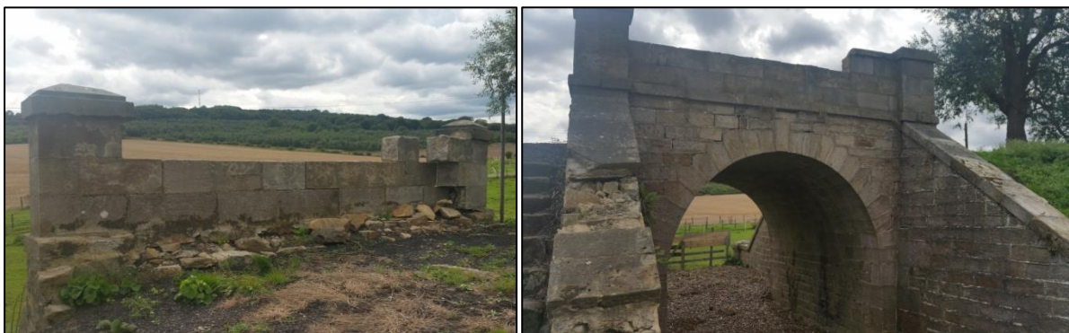
Plate 9. Brusselton Accommodation Bridge, showing recent vandalism and stone theft to parapet and water tabling.
