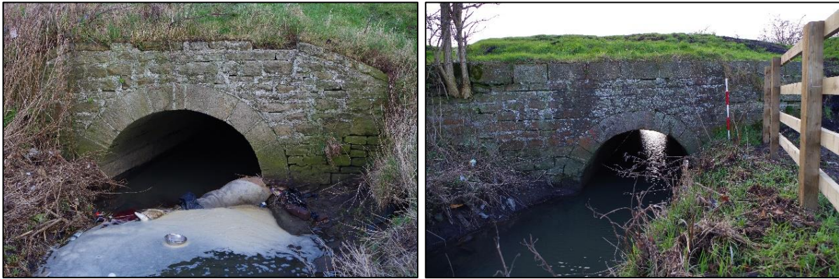
Plate 1. Original 1825 culvert; viewed from below the railway embankment on the south side (left) and the north side (right)
