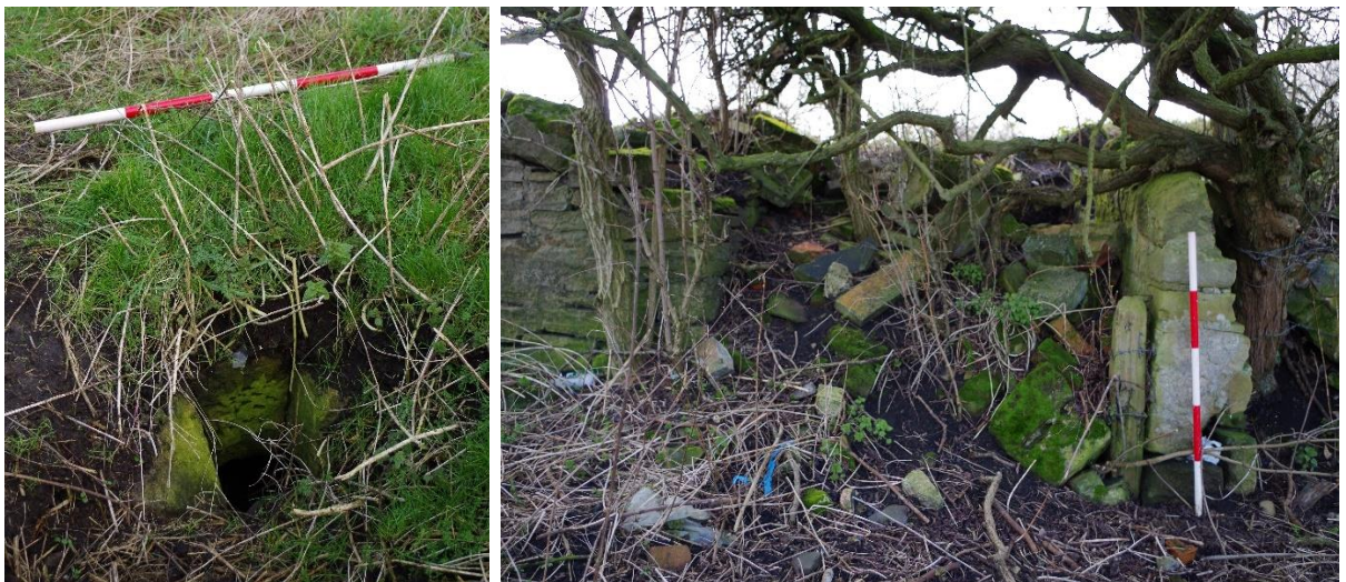
Plate 4. Both sides of the buried accommodation bridge now buried beneath the embankment
