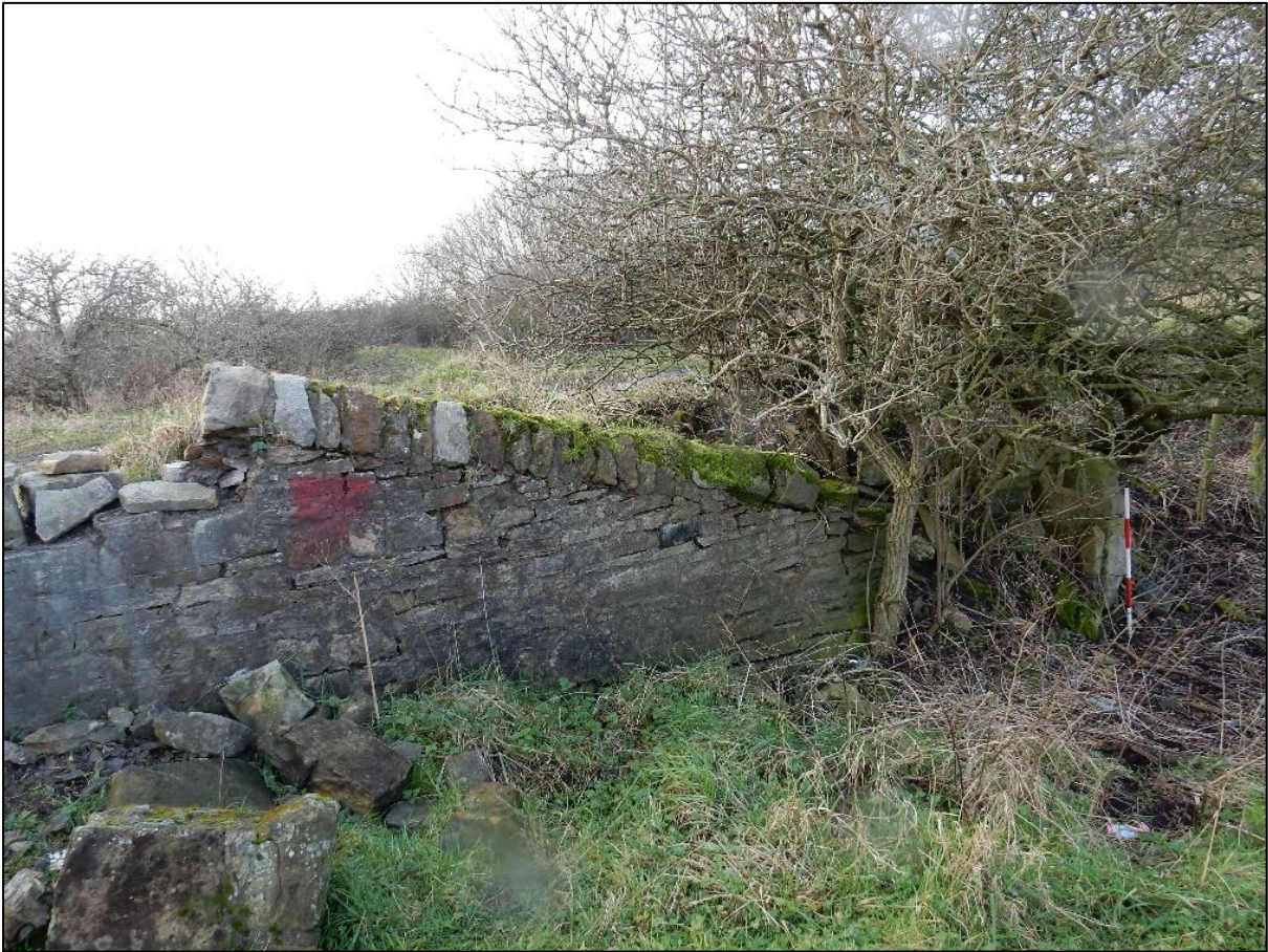
Plate 3. Sloping boundary wall indicating an adjacent structure – in this case a long forgotten and buried accommodation bridge and ramp
