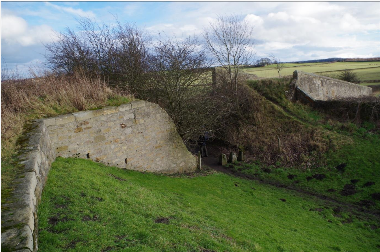
Plate 18. The imposing remains of the Milk Bridge on the eastern side of Brusselton Incline. An original structure currently with no legal protection other than being in a conservation area.
