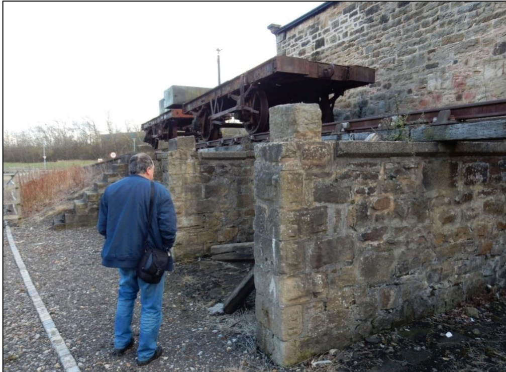
Plate 10. The elevated ramp to the rear for dropping coal into waiting carts for domestic sale, known as 'landsale' (as opposed to being taken to the port for export known as seacoal)
