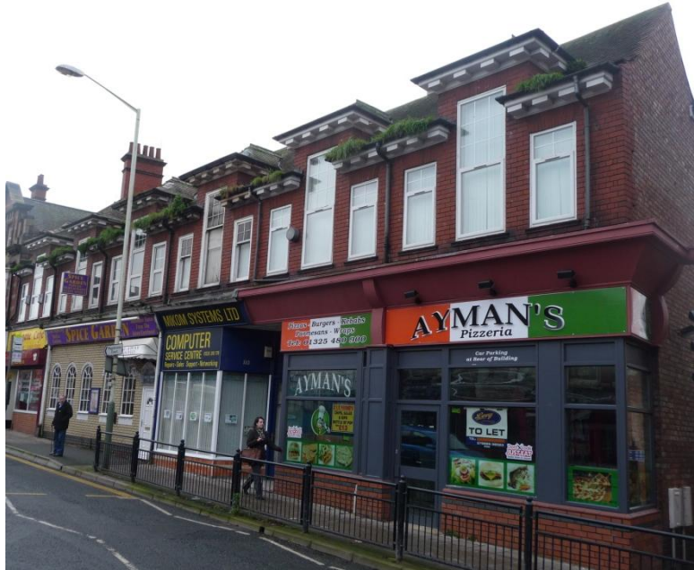
Plate 20. This building displays a number of management issues. Grass is growing from the gutters, a shop front has been reclad in inappropriate materials which along with garish and overly large fascias breaks up the unity of design at ground floor level
