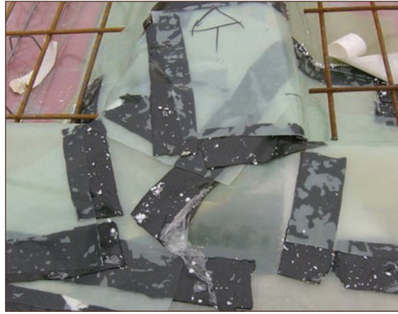
Figure A4.68 A pre-formed corner unit would have been preferable. The installer could not produce sufficient quality despite the amount of tape applied (courtesy Smith Grant)
