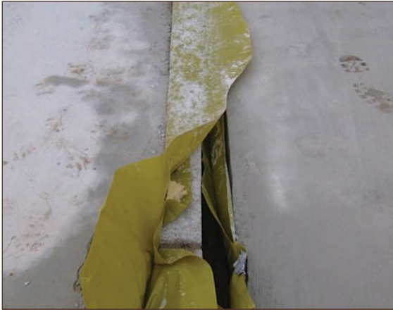
Figure A4.79 Gas membrane not continuous over internal wall. It had been deliberately cut open for unknown purpose (courtesy Smith Grant)
