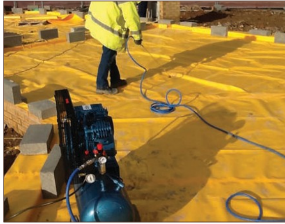
Figure A4.44 Air lance test, used to test the quality of welded seams along gas membrane joints (courtesy MEC Environmental Ltd)
