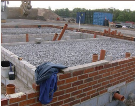
Figure A4.85 Clean single sized stones with no fines acting as venting media, however no ventilation gaps in internal sleeper walls (courtesy Smith Grant)
