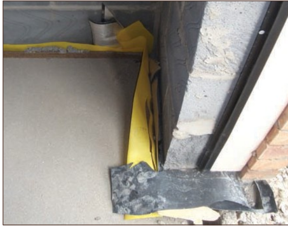
Figure A4.70 Inadequate corner detailing. The use of preformed proprietary products would have avoided such bad practice (courtesy NHBC)
