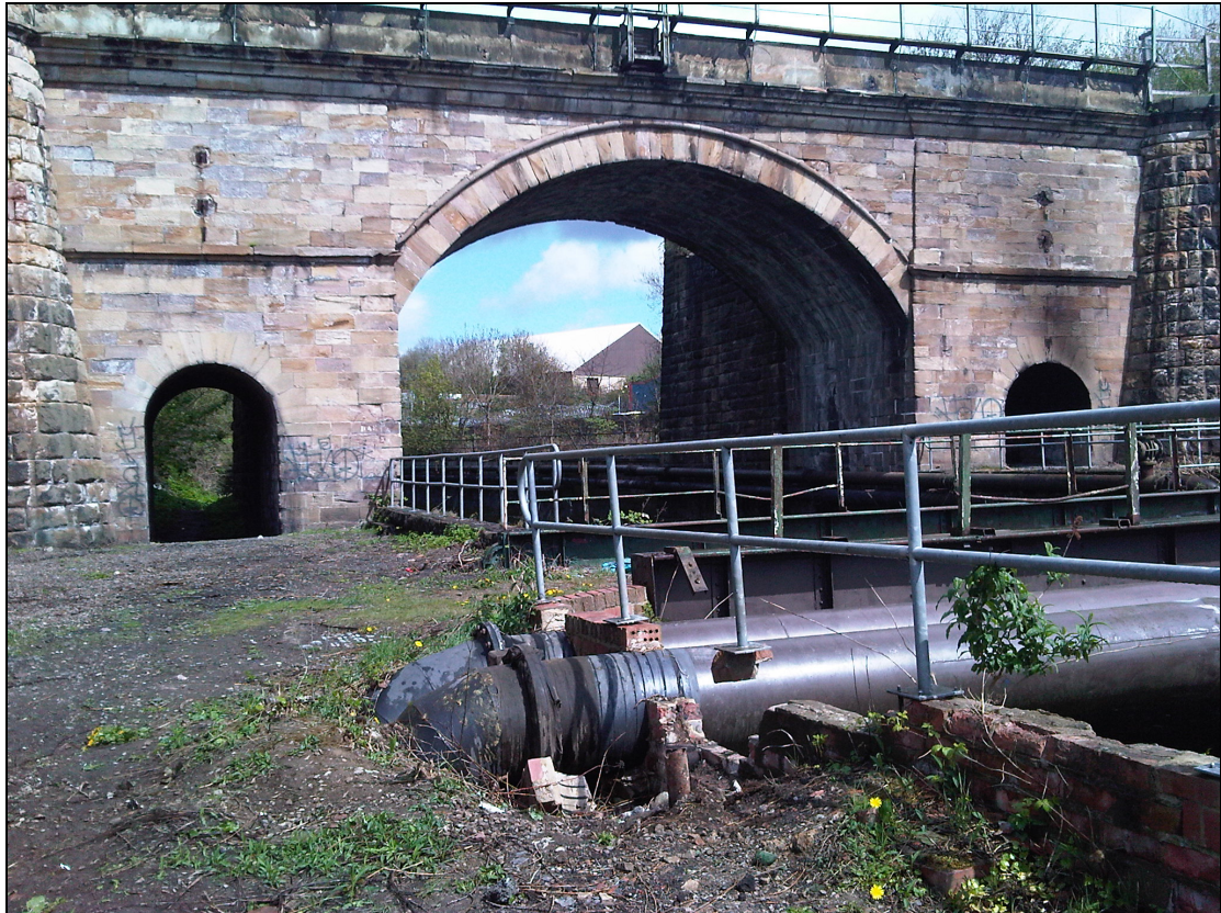
Plate 43. The Skerne Bridge, also known as the five pound note bridge. The setting of this scheduled monument has been marred by the gas pipes, railings and poor access which limits the experience of the bridge
