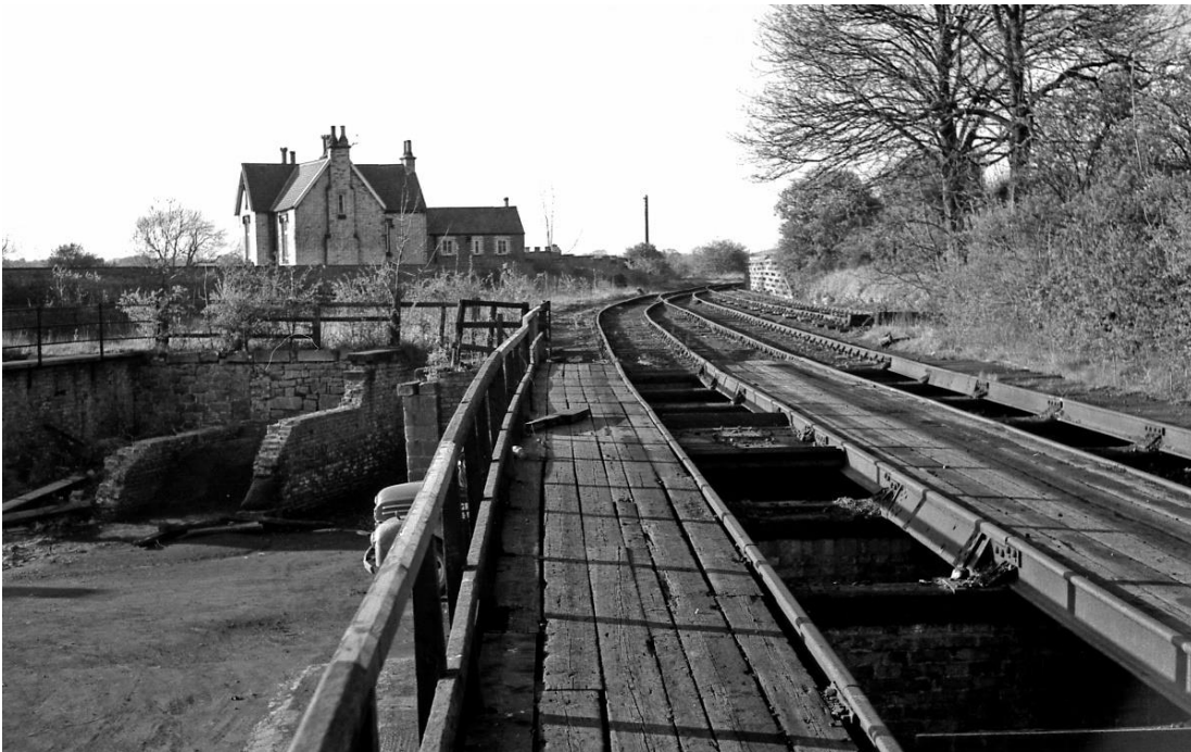
Figure 72. The top of the coal drops where coal was dropped into cells below from wagons on the higher trackbed. The wooden platforms on either side of the drops were for depot attendants to stand and help unload the wagons. More cells to the left have lost their overhead tracks. Image dated 1964. (Photo R. V. Webster).
