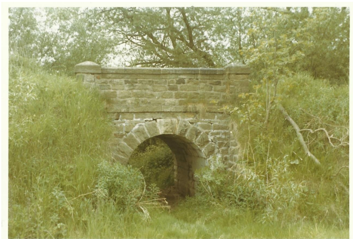
Figure 61. Railway bridge near Croft in 1971 (not seen during incomplete site visit) (photo: John Proud)
