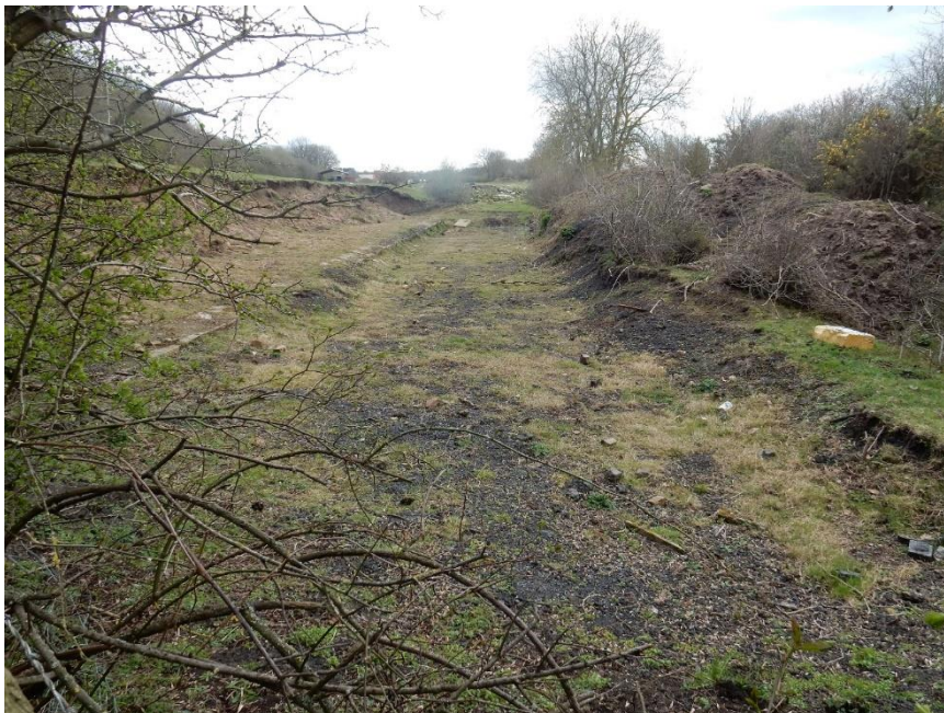
Figure 52. The cutting as it levels towards Black Banks. Stone revetments can be seen on the left side and these presumably continue to the south but are buried by woodland vegetation. The embankments to the left seem to be subject to quarrying for soil.
