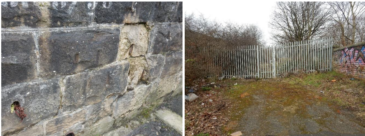
Figure 34. Left: reused and split two hole sleeper blocks from the 1829 trackbed incorporated into pre 1855 stonework. Right: a later 19 th c cattle ramp giving a livestock route on to the cattle pend and sidings
