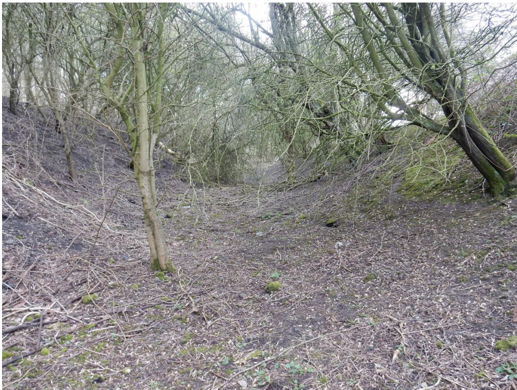
Figure 50. The cutting for the Croft trackbed just south of the A66 and north of Black Banks.
